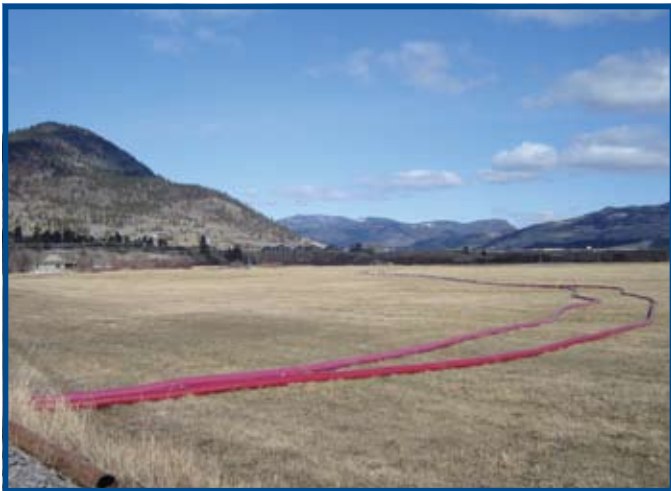
Figure 8. Discharge pipe for a large volume pumping test in Merritt.
