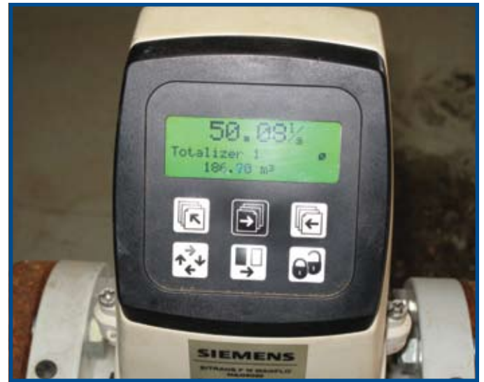
Figure 4. In-line flow meter.
